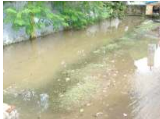
Choked drain causing water logging
