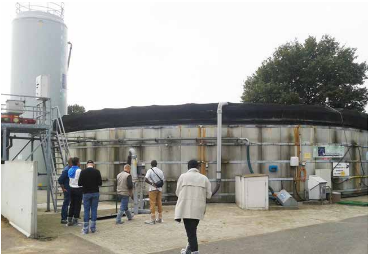
Biogas reactor in the Netherlands. Photo: René van Veenhuizen
